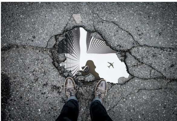
Potholes caused by wear and tear
